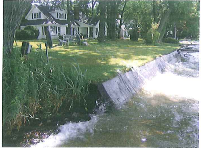
Figure 2.6. Waves flanking off neighboring seawall. (Photo: Jane Herbert.)
