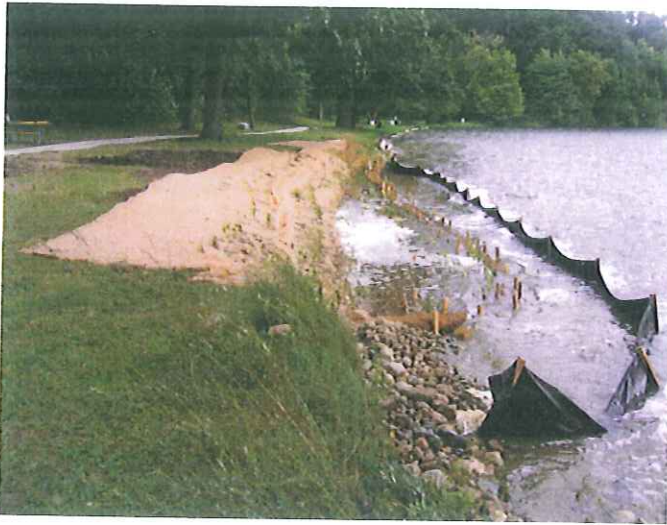
Figure 4.14. Coir logs of insufficient diameter are overtopped by waves, which then disturb nearshore aquatic plantings. (Photo: Jane Herbert.)
