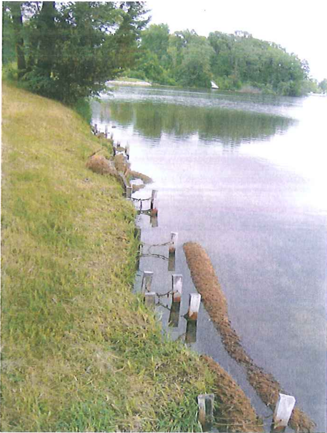
Figure 6.2. Poorly maintained coir logs can become a navigational hazard when displaced by wave action. (Photo: Jane Herbert.)
